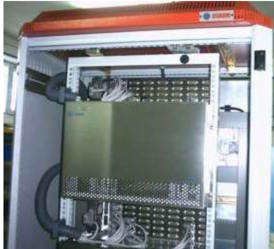
Figure 4 Uskom Multiplexer System in Al Ameen S/S, Iraq
