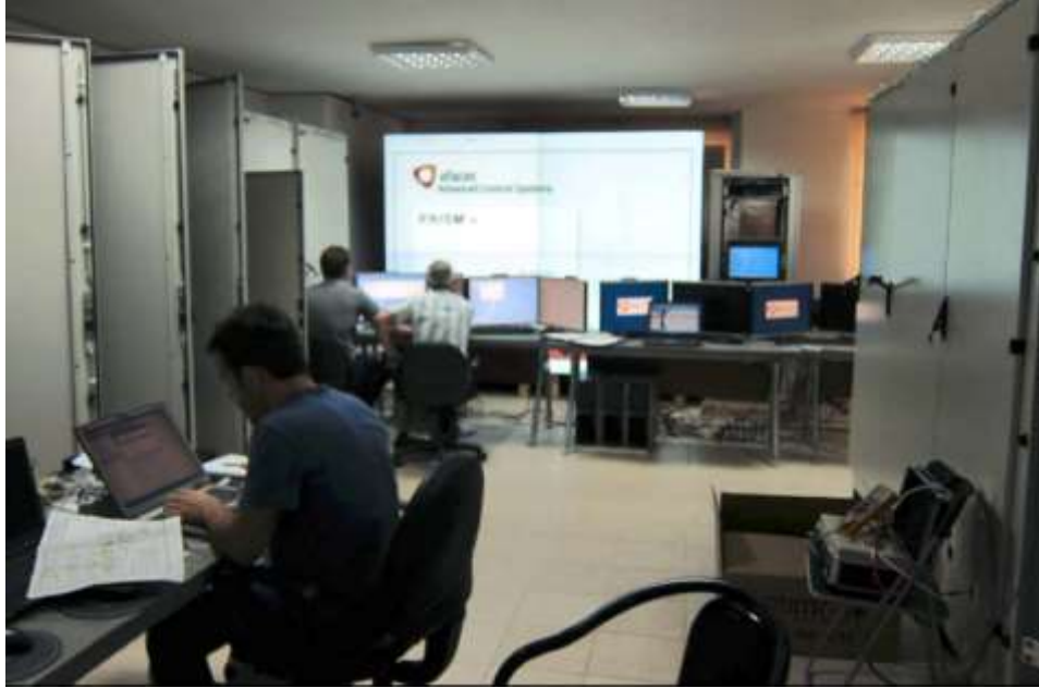
Figure 2 Uskom FAT Hall, FAT for LBGBV National SCADA Load Control Center
