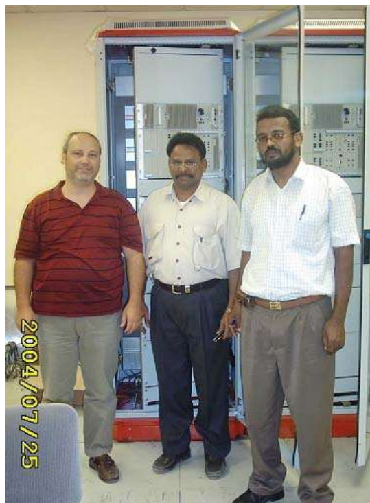
Figure 1 Uskom PLC System in Saudi Arabia
