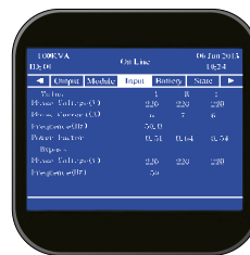
UPS Kabin Kontrol Paneli
